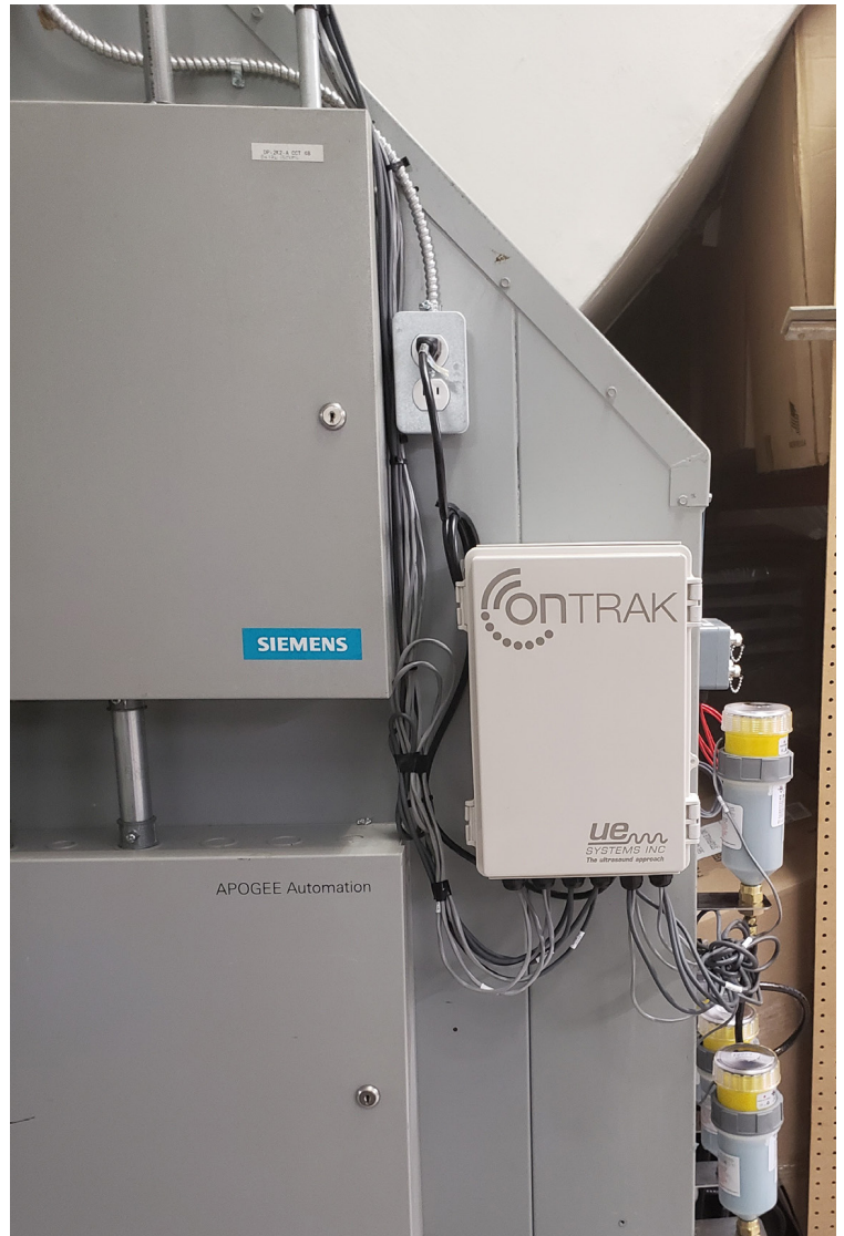
OnTrak System Gathering Data from Sensors on AHUs
