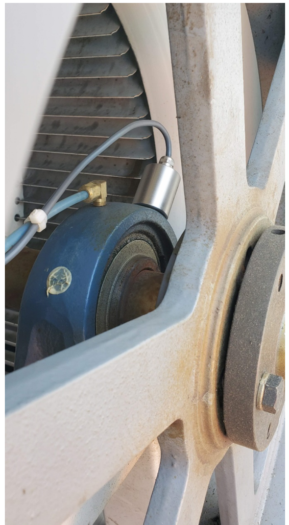
OnTrak Sensor Installed on AHU
