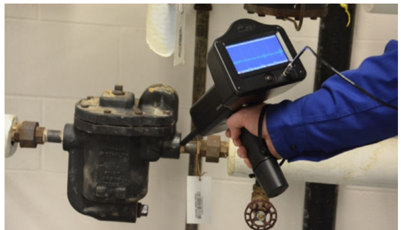
Figure 2 Inspector performing steam trap inspection on plant steam system using the UE Systems Ultraprobe.
