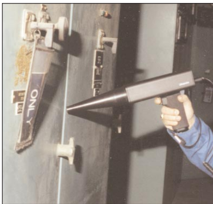
Figure 5. Arcing, tracking, corona, and partial discharge produce ionization. Inspectors can identify the type of problem based on the sound patterns. Enclosed systems can be tested by scanning door seams and air vents. A contact probe can be used on totally enclosed systems.
