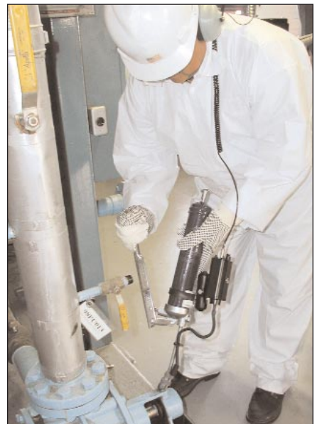
Figure 4. Overlubrication is one of the most common causes of bearing failure. To prevent this, when bearings are identified for lubrication, technicians can use ultrasonic translators to listen while the lubricant is applied and recognize when to stop lubricating.
