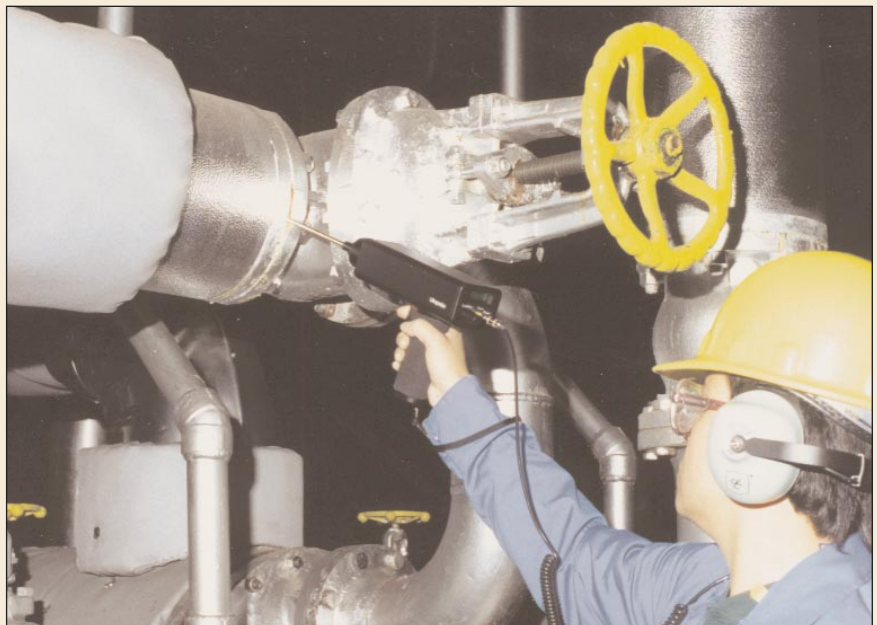
Figure 1. Ultrasound is a localized signal that makes detecting a leaking valve relatively easy. Sound levels are compared upstream vs. downstream. A louder downstream sound will indicate a leak.
