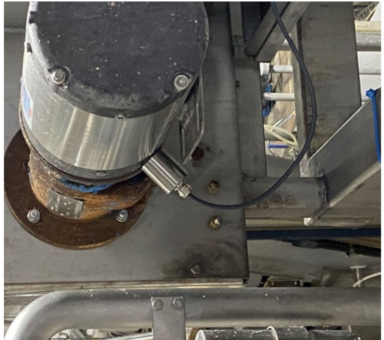
Figure 2. OnTrak system installed
